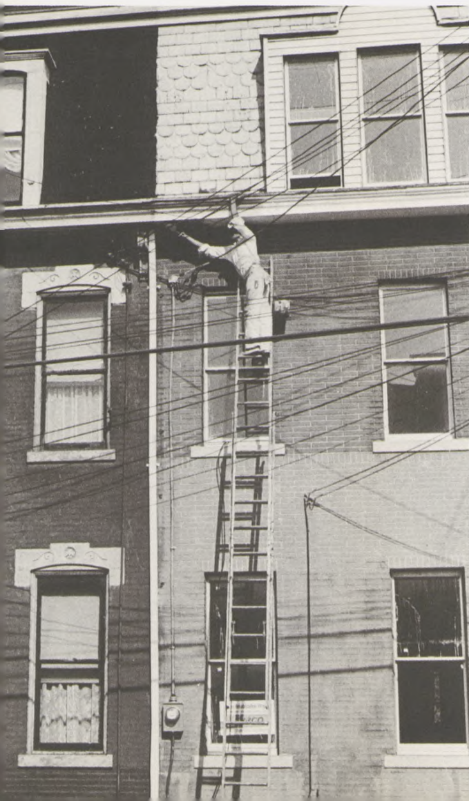
Rehabilitation of old but structurally-sound housing, such as these two homes in Pittsburgh's Hill District, is the business of AHRCO.
