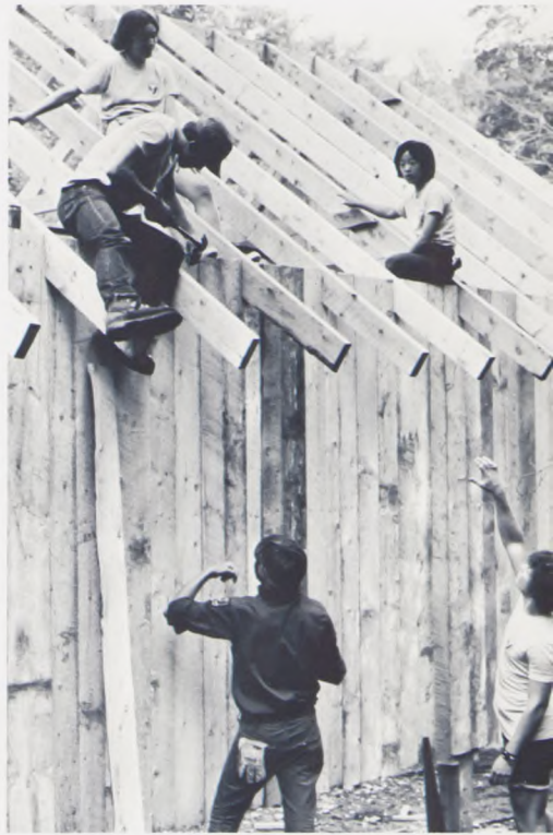
High school and college students in the Student Conservation Association's programs provide the manpower to build needed facilities in our national parks.
