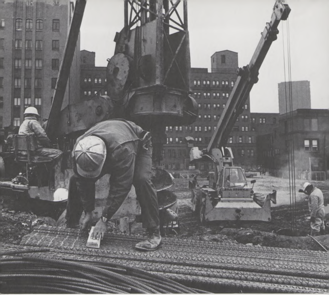
New hospital site: with the excavation nearly completed, foundation work for the new Mercy Hospital gets underway. Parts of the old Mercy complex can be seen in the background.
